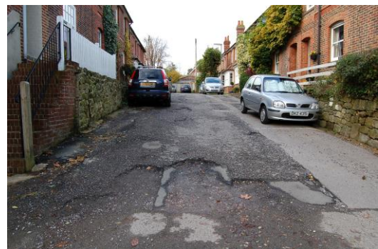
Figure 22: Road surface at Northfields
